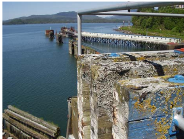
Figure 5. Ferry terminal overhead beams exposed to sun and rain
