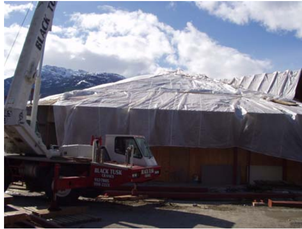
Figure 1. Temporary tarps over architectural grade glue-laminated beams
