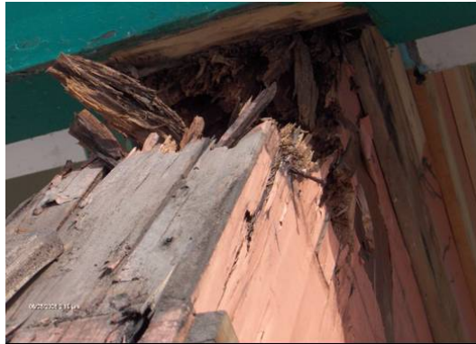
Figure 3. Neglected, untreated arch suffering rot through one-third of its depth
