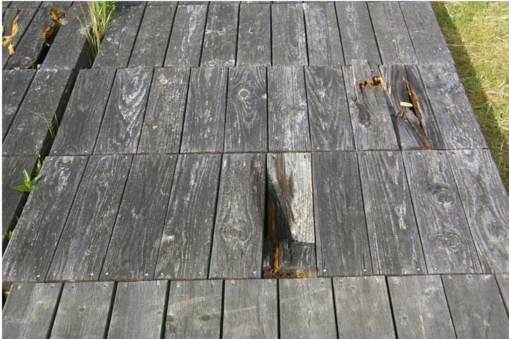
Figure 4: Southern pine untreated deck in Vancouver
