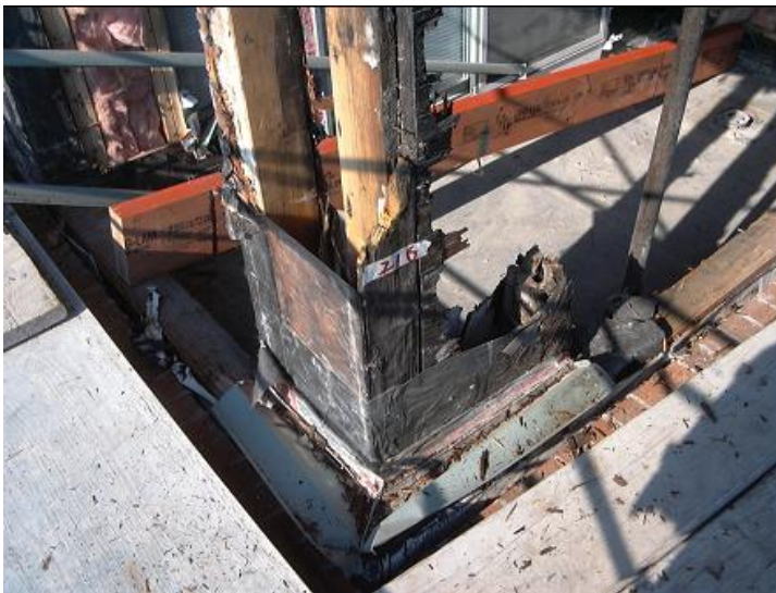
Photograph 1: Decayed balcony column.
