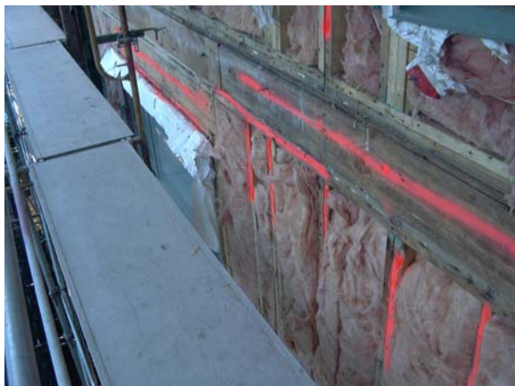
Photograph 4: Wood framing marked for replacement.
