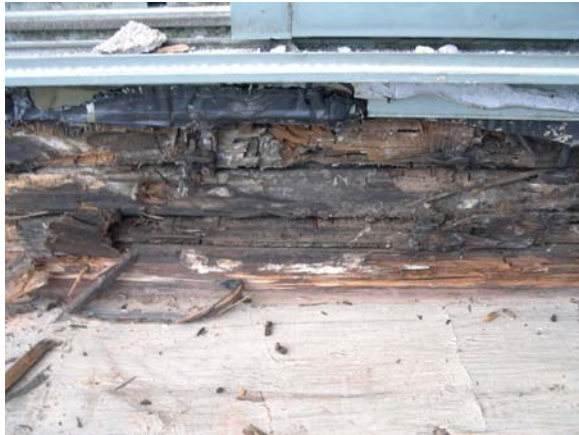
Photograph 2: Decayed sill plate.
