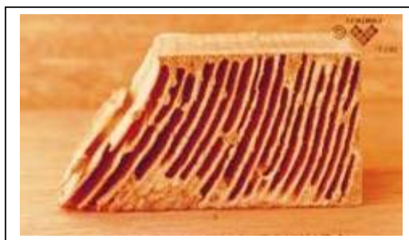
Fig. 4 Wood damaged by subterranean termites.
