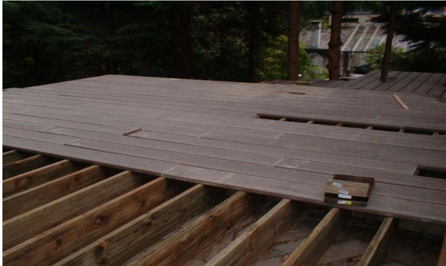
Figure 3.7 - Photo of my deck under construction – 2x12 ACQ treated beams, 6x6 ACQ treated posts, 2x10 ACQ treated joists, and 2x10 Trex Decking.
