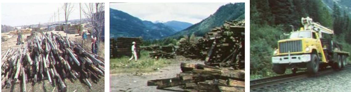
Figure 11: Out of service poles and ties and truck for collection of removed ties
