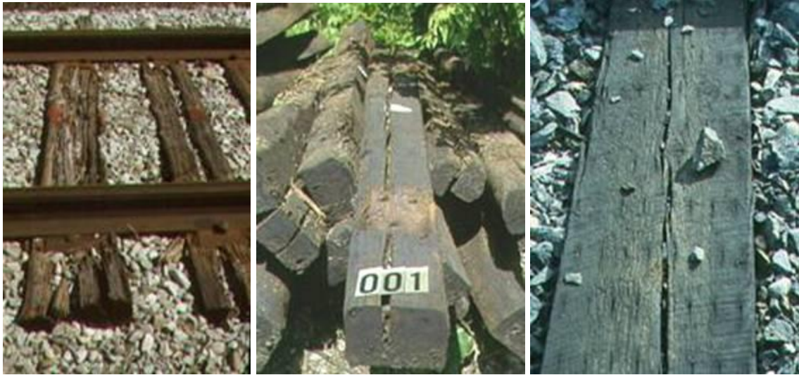
Figure 15: Splitting and other defects in ties and role of ballast stones in splitting
