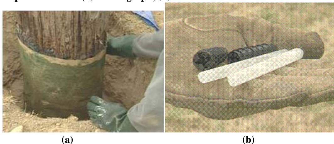
Remedial Treatments (a) Surface pole wrap (b) diffusing borate rods for internal treatment Figure 4: Pole inspection and pole treatment processes
