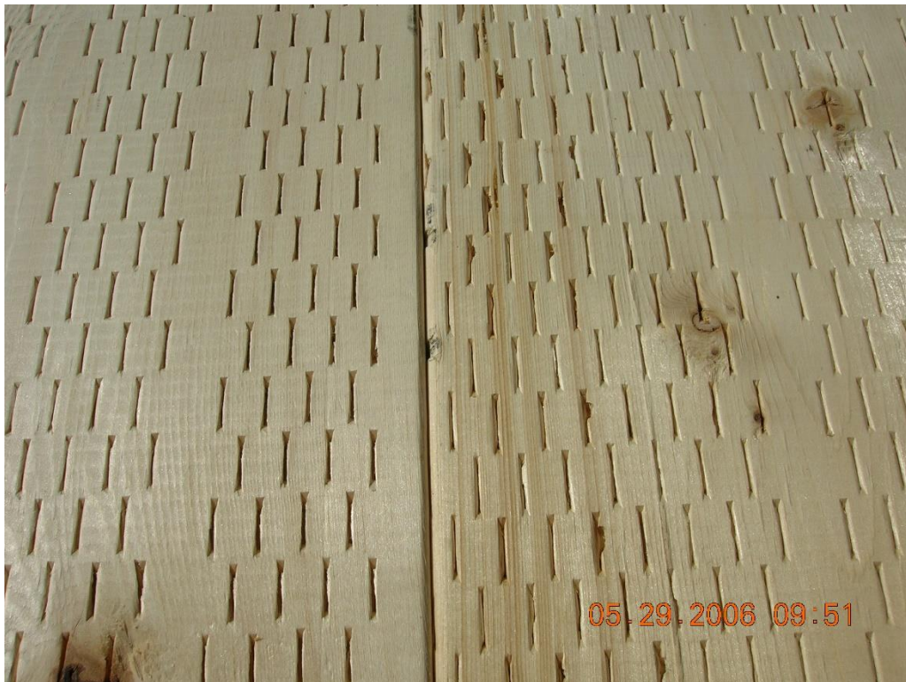
Photo 1: Spacing Gaps on the Surface of WWP Incised 2x8 Western SPF
