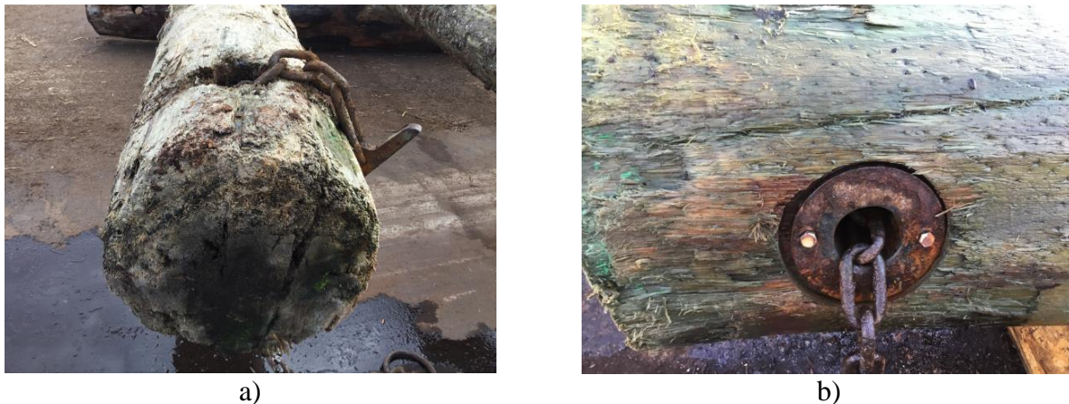
Figure 7. Mechanical damage observed in control sticks (a) and treated sticks (b)
